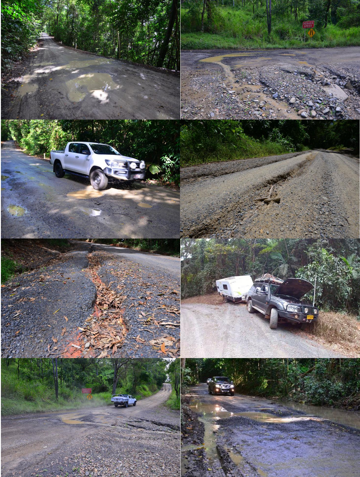
Photos #4: Rough road surface slow traffic result in higher operating costs
